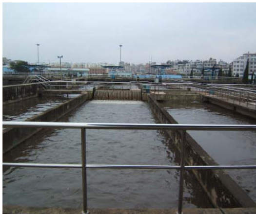
Biological treatment unit (Bardenpho) WWTP No. 1
