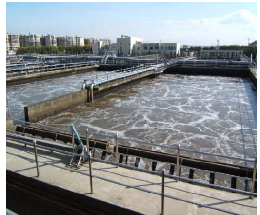
Biological treatment unit (ICEAS) WWTP No. 3
