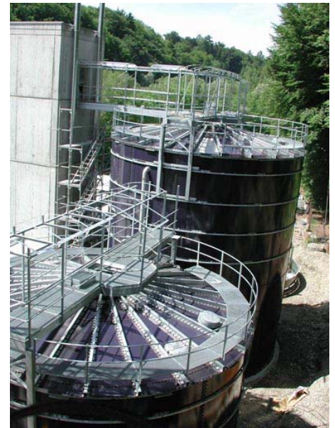
Picture right: New building of the secondary thickener and of the premises for this part of the installation. Most advanced technics is combined with existing parts of the installation.
