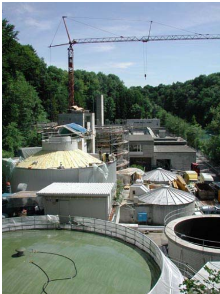
Picture left: Sanitation of the existing sludge processing. During the modification phase the works are in that way coordinated, that the line operation (in a reduction availability) is ensured anytime.
