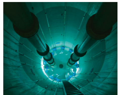
Drinking water well in the Töss Valley in vicinity of the river (Source: Stadtwerk Winterthur)
