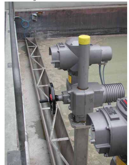
Picture right: New, fully automatic extraction of the floating sludge of the primary sedimentation basin
