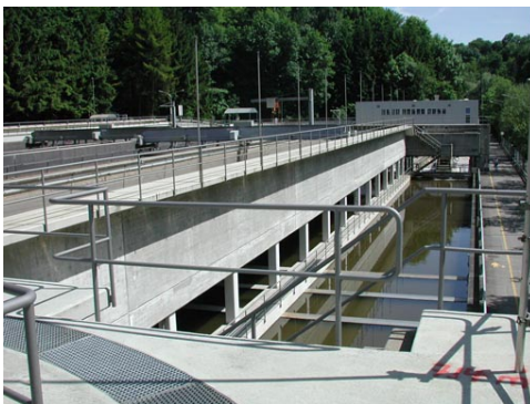
Picture left: Existing biological purification stage with primary sedimentation basin (left), aeration tank (background) and secondary sedimentation basin (right)
