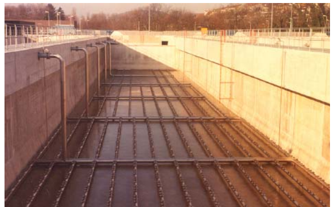
Aeration tanks with fine bubble aeration system for activated sludge treatment system
