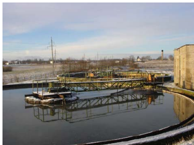
Final clarification of biological treatment unit
