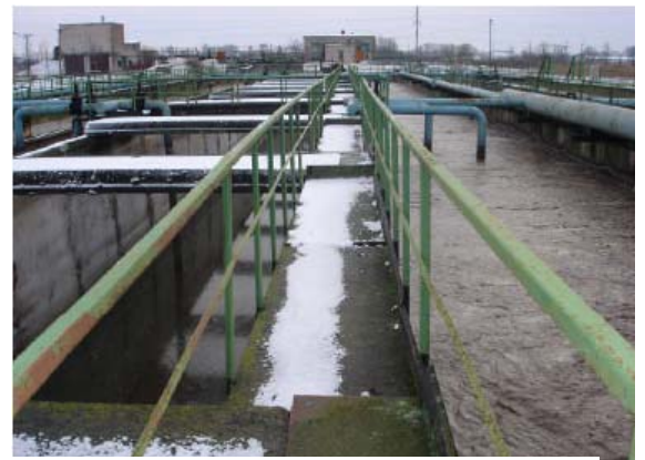
Biological treatment unit with activated sludge
