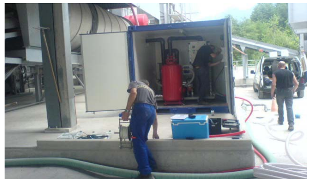
Installation de bioventing
