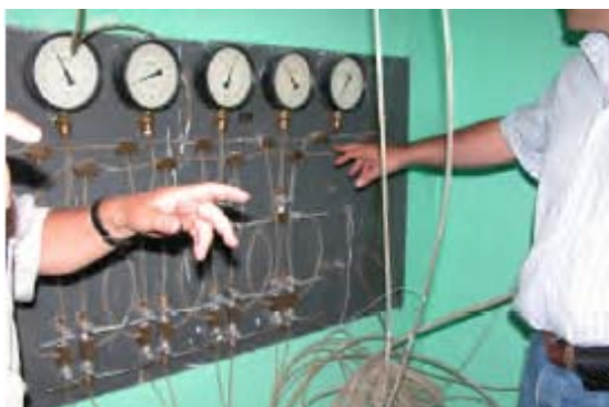
Pore pressure monitoring at Vaut I Dejes Dam
